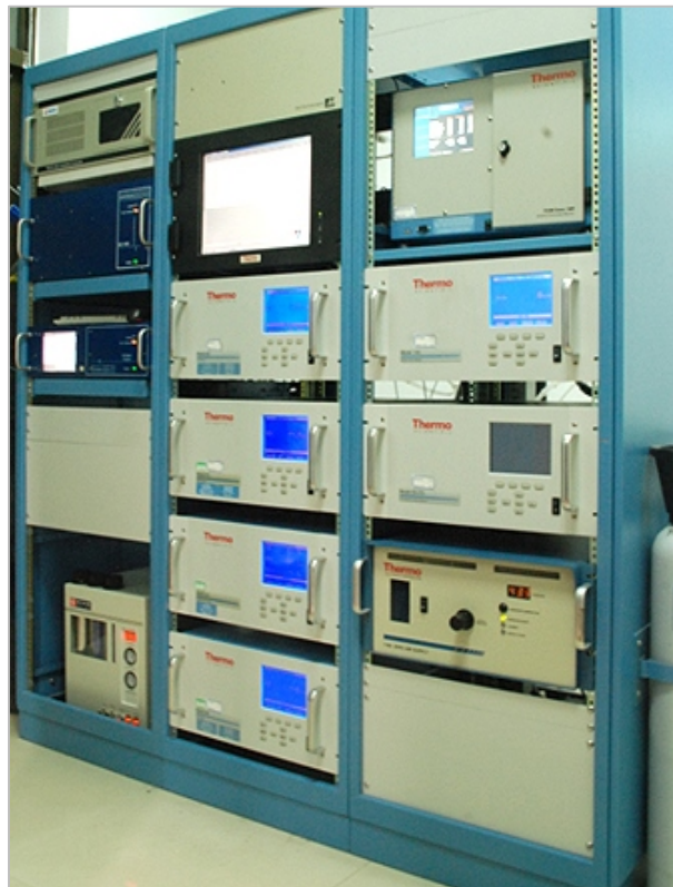
FIGURE 4 EXAMPLE OF RACK-TYPE ANALYZER MOUNTING WITHIN A SHELTER
